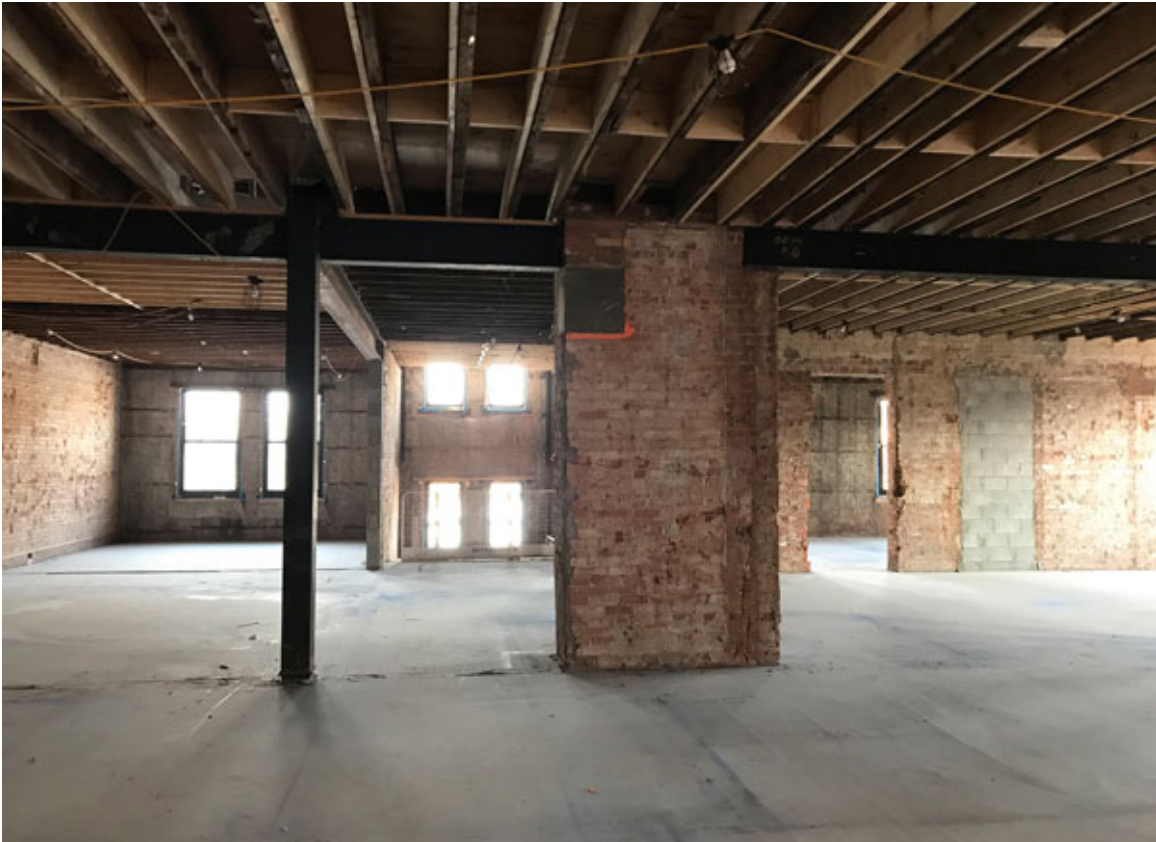
PHOTO SUBMITTED — Creating the Y Lofts was a challenge, state the developers, with asbestos discovered, along with mold and lead paint. Every wall had to be sampled and stripped down.
